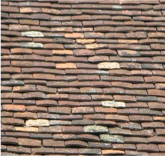
A second hand peg tile roof in the South East, showing the variety and age of tiles which might occur including yellow gault tile.
